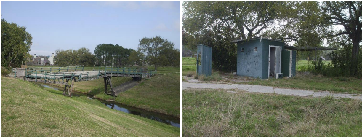
Images of aging infrastructure, bridge (above left) and restroom (above right), at the defunct golf course
